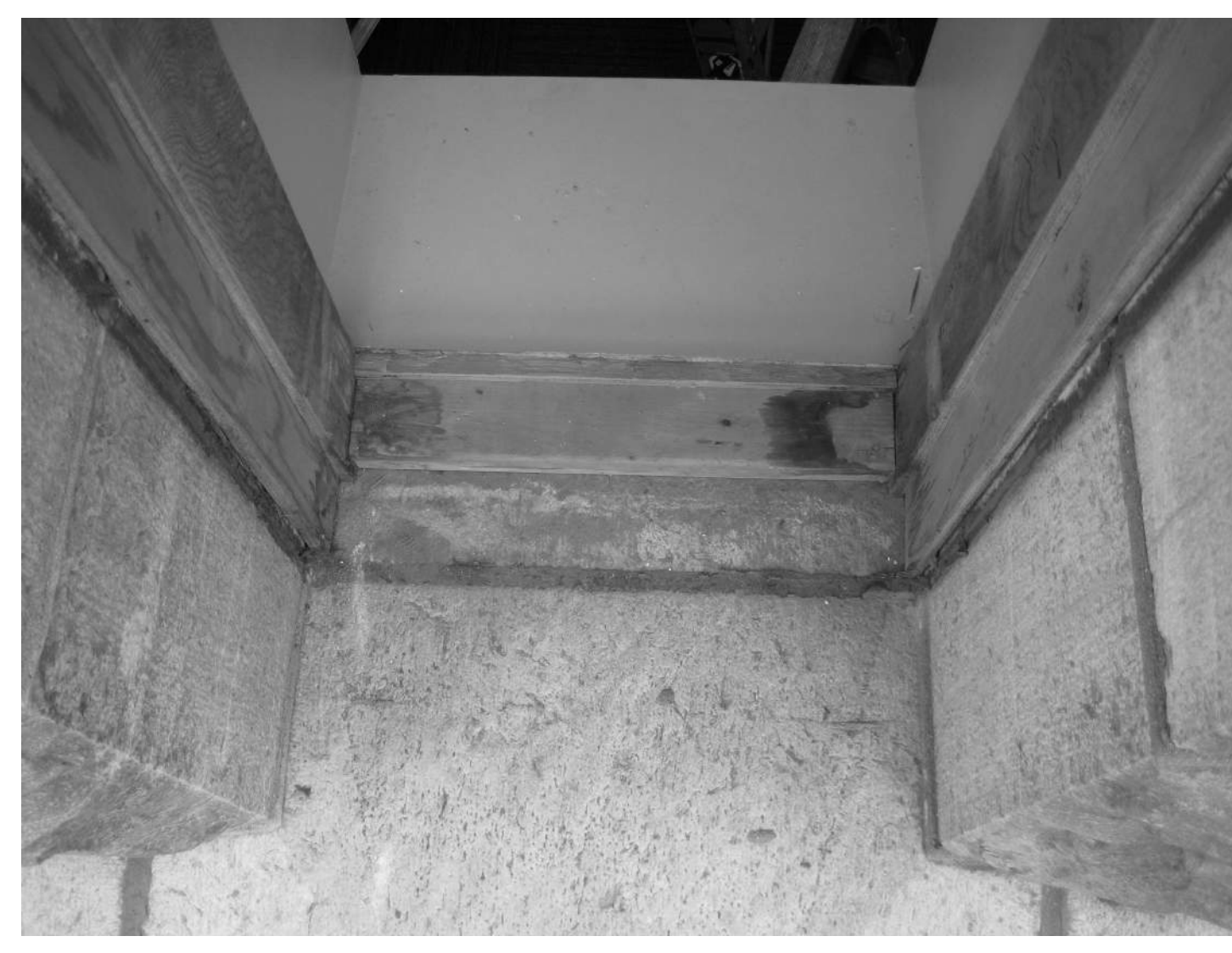
21 FIRST FLOOR WINDOW DEMO SILL CONDITION - AT WEST ELEVATION SCALE: 3" = 1'-0"
