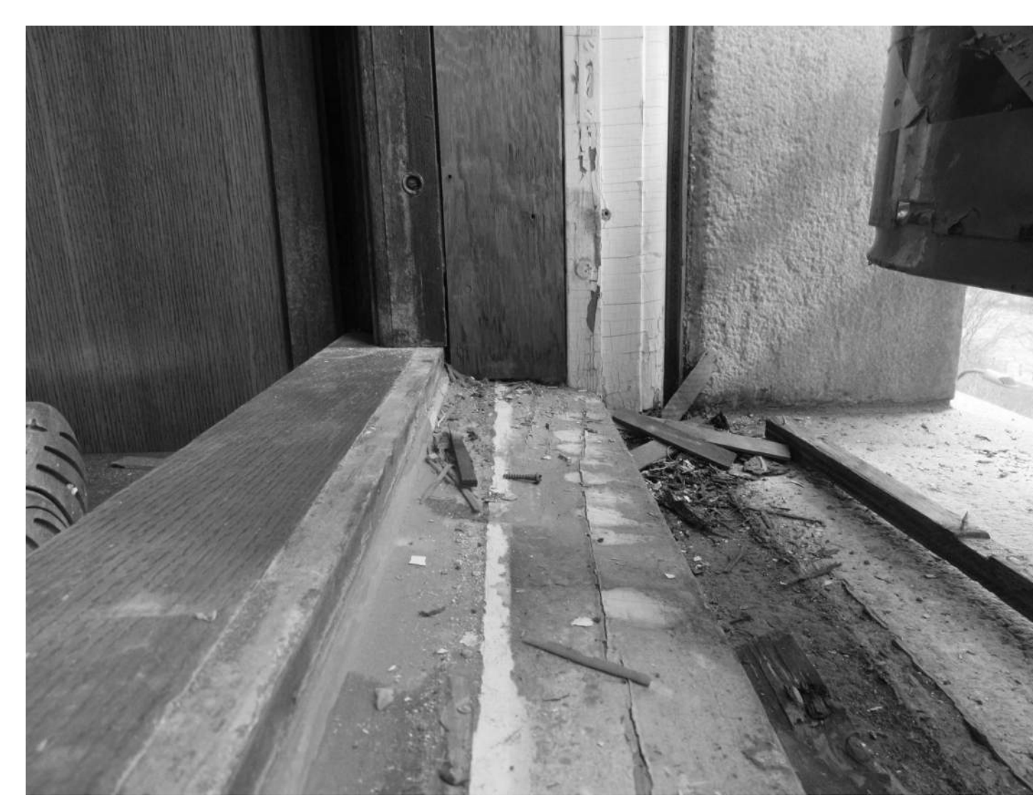
34 SECOND FLOOR WINDOW DEMO SILL CONDITION - AT EAST ELEVATION SCALE: 3" = 1'-0"
