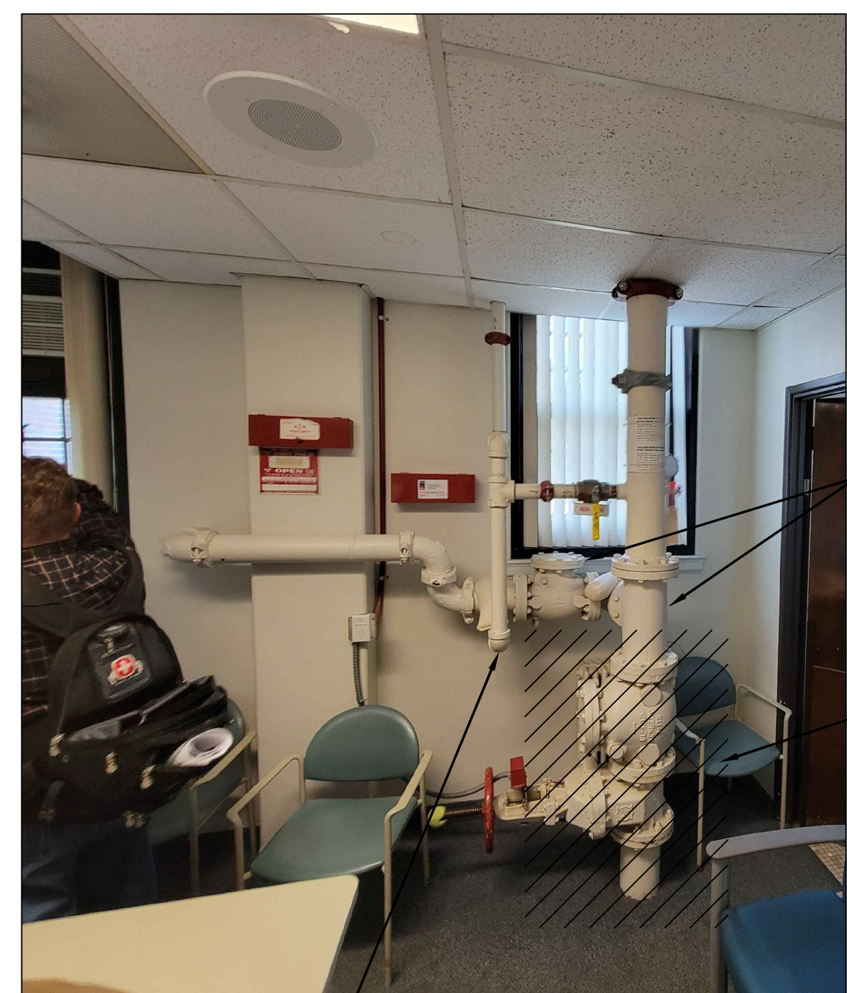
CONTRACTOR TO VERIFY EXISTING DRAIN IS SUFFICIENT FOR TESTING OF SYSTEM
