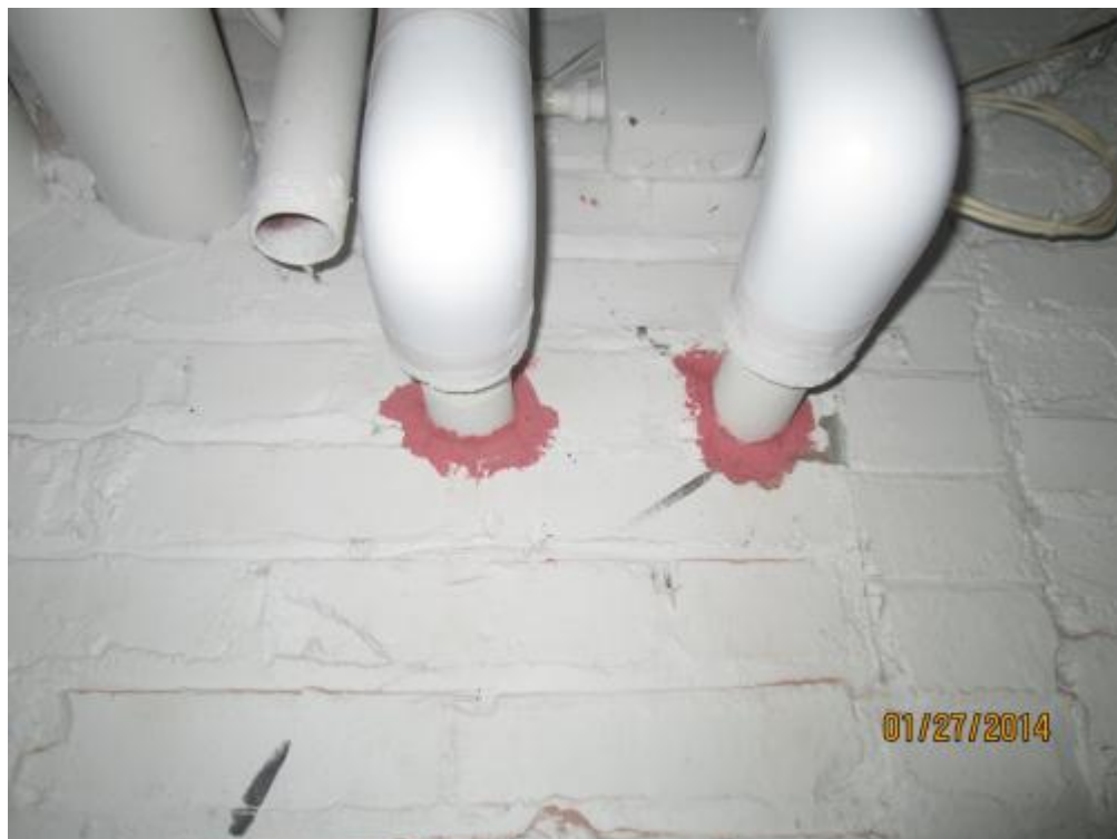
PPS01 – Pipe Penetration Sealant – pink (No Asbestos Detected).
