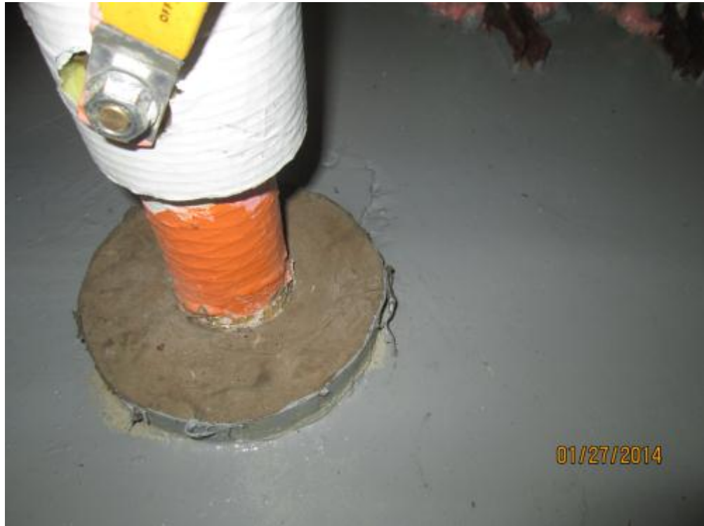
PPS02 – Pipe Penetration Sealant – light brown and painted green (No Asbestos Detected).
