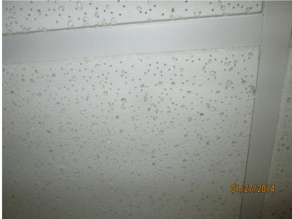
CT01 – Ceiling Tile – 2'x2' white with dots and small fissures (No Asbestos Detected).
