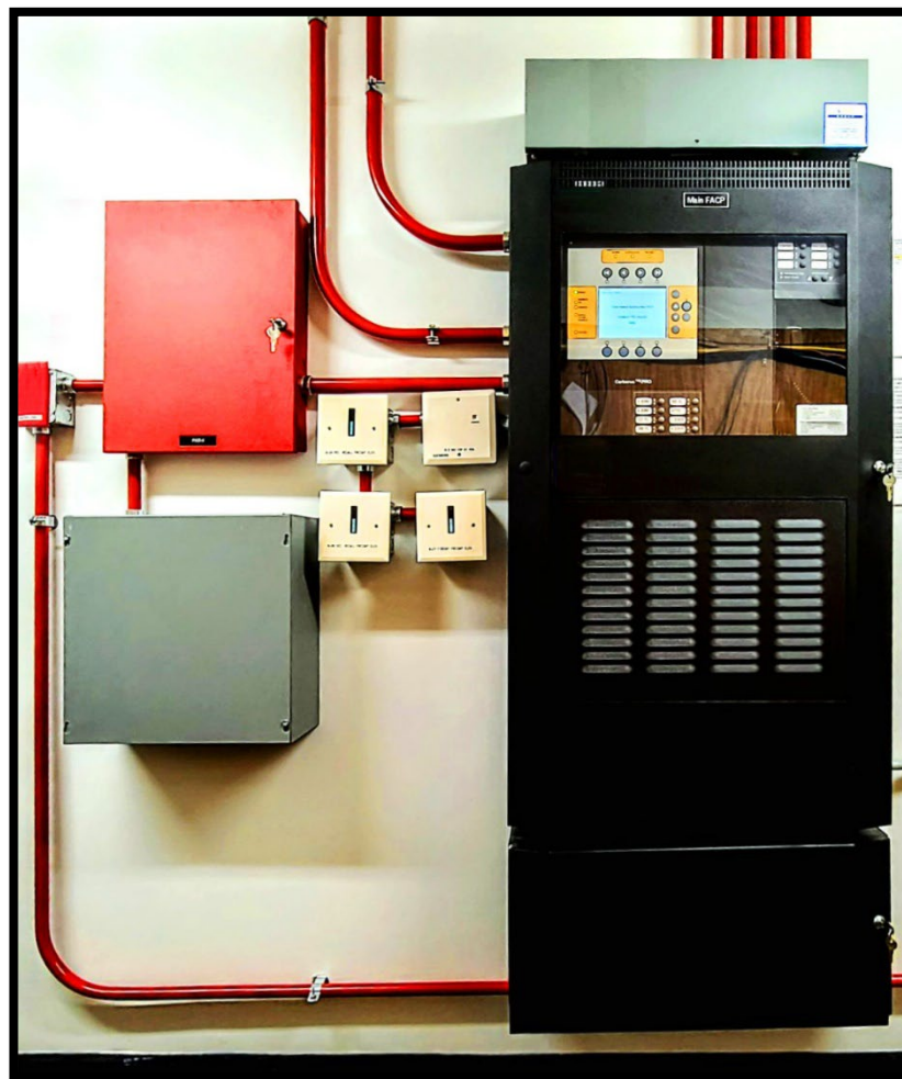
Figure 20: National Support Center Social Security Administration Fire Panel Woodlawn, MD
