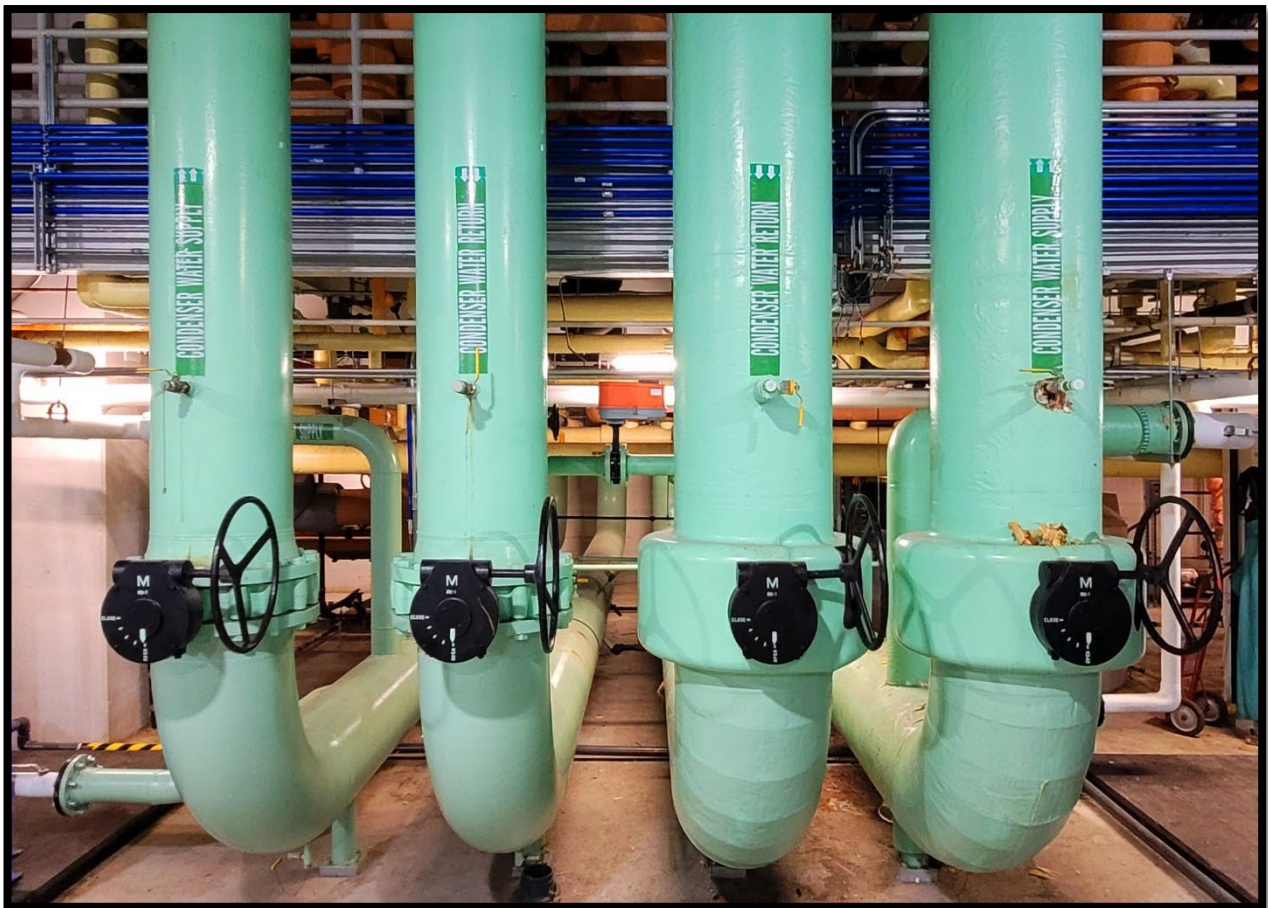
Figure 16: Ronald Reagan Federal Building Mechanical Piping Washington, DC
