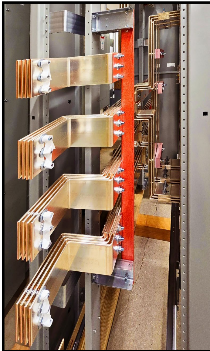
Figure 18: Building 48 Denver Federal Center Electrical Denver, CO
