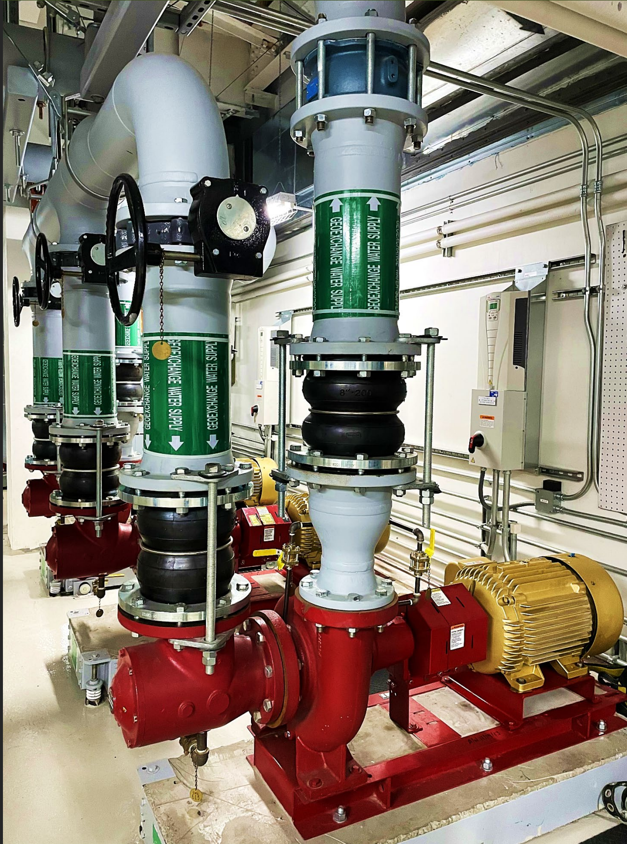
Figure 15: Land Port of Entry Geothermal System San Ysidro, CA
