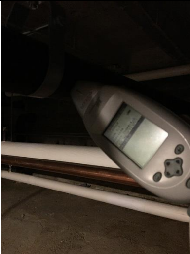
PHOTO 35 Black Pipe – Tunnel <1mg/cm 2 lead
