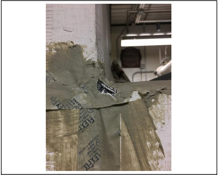
PHOTO 2 Gray Mastic – Duct in below grade mechanical room
