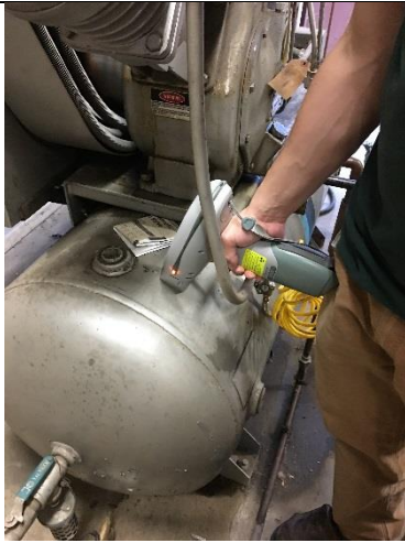
PHOTO 7 Silver Painted Tank – Below Grade Mech. Room <1mg/cm 2 lead
