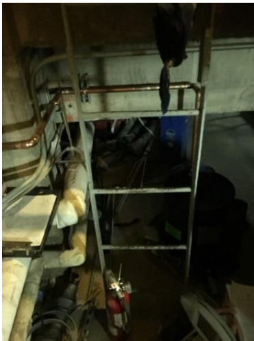
PHOTO 41 Gray ladder in Tunnel 3.1 mg/cm 2 lead
