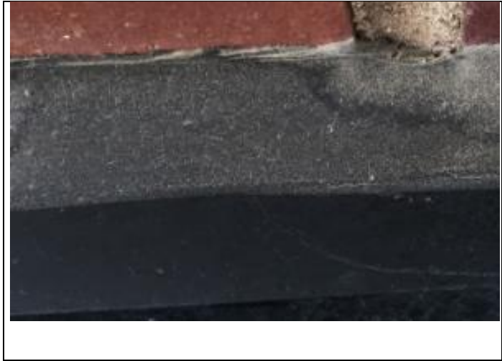
PHOTO 11 | Gray Window Caulk - Exterior
