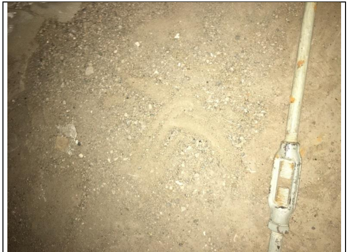
PHOTO 16 Debris on Tunnel Floor
