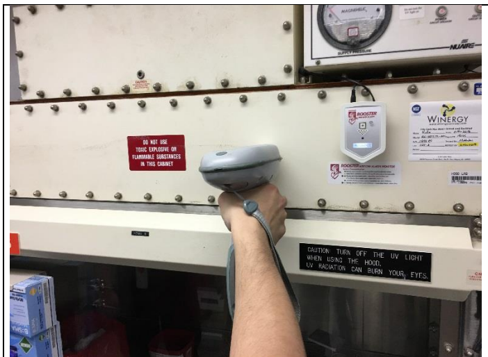
PHOTO 69 Cream Fume Hood – West Wall <1mg/cm 2 lead
