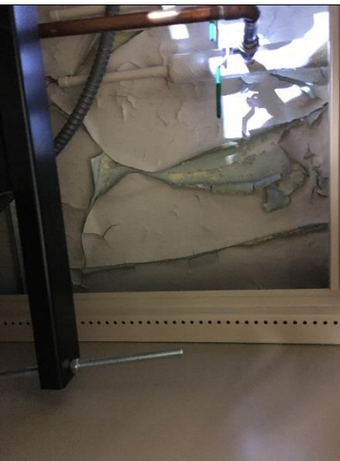
PHOTO 75 Peeling White Paint Under Sink <1mg/cm 2 lead
