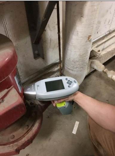
PHOTO 11 Red Painted Mixing Chamber – Below Grade Mech. Room <1mg/cm 2 lead
