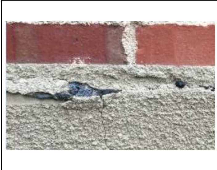
PHOTO 7 | Black Tar Under EFIS – Mech. Room Entry
