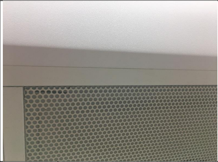
PHOTO 55 Ceiling Grid Hallway by D-17 <1mg/cm 2 lead
