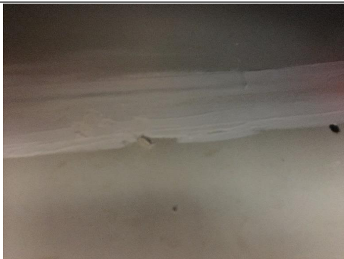
PHOTO 21 | Drywall/Joint Compound D-17
