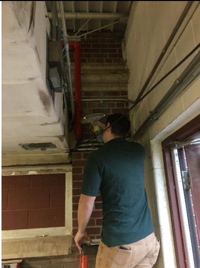
PHOTO 15 Red Painted Pipe – Below Grade Mech. Room <math><1\text{mg}/\text{cm}^2\text{ lead}</math>
