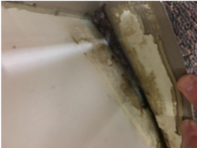
PHOTO 25 Tan Base Cove Mastic
