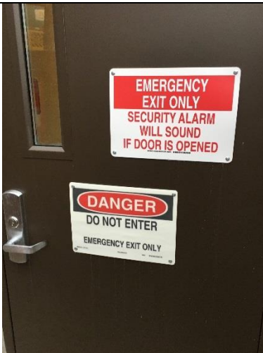
PHOTO 23 Brown Door (Outside) <1mg/cm 2 lead
