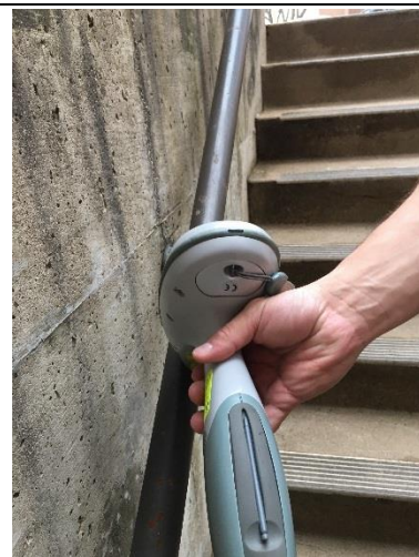
PHOTO 24 Brown Hand Railing-Stairs to Mech. Room 1.7 mg/cm 2 lead
