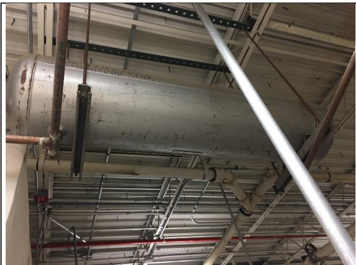
PHOTO 18 Silver Overhead Tank – Below Grade Mech. Room <math><1\text{mg}/\text{cm}^2\text{ lead}</math>
