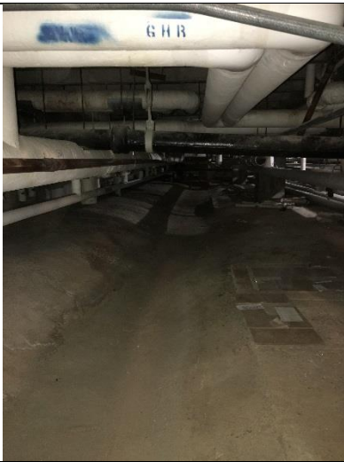
PHOTO 34 Black Pipe – Tunnel <1mg/cm 2 lead
