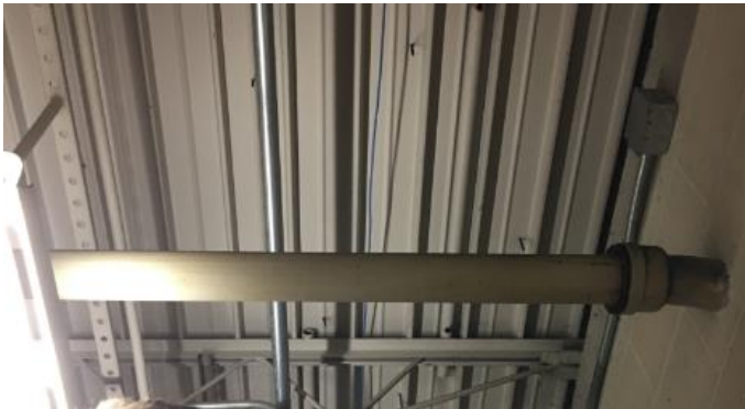
PHOTO 17 White Painted Pipe – Below Grade Mech. Room <math><1\text{mg}/\text{cm}^2\text{ lead}</math>
