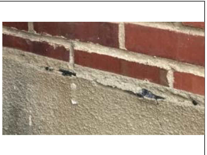
PHOTO 6 Black Tar Under EFIS – Mech. Room Entry
