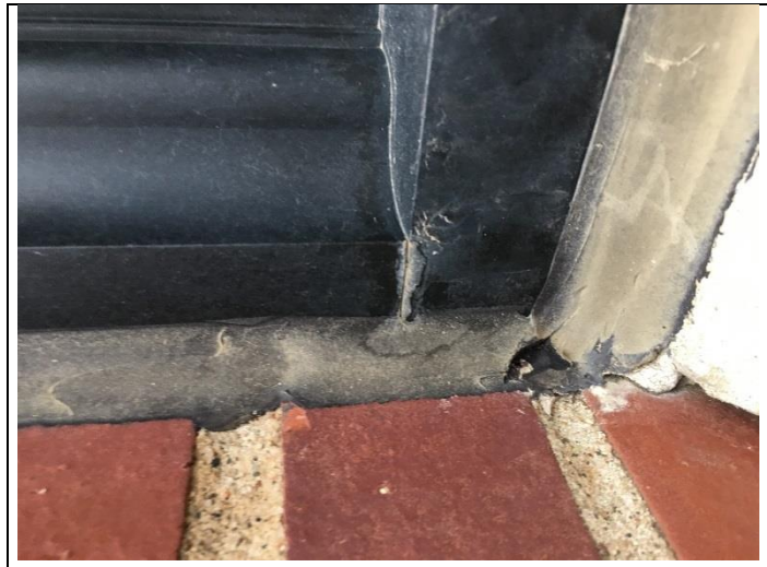
PHOTO 10 | Gray Window Caulk - Exterior
