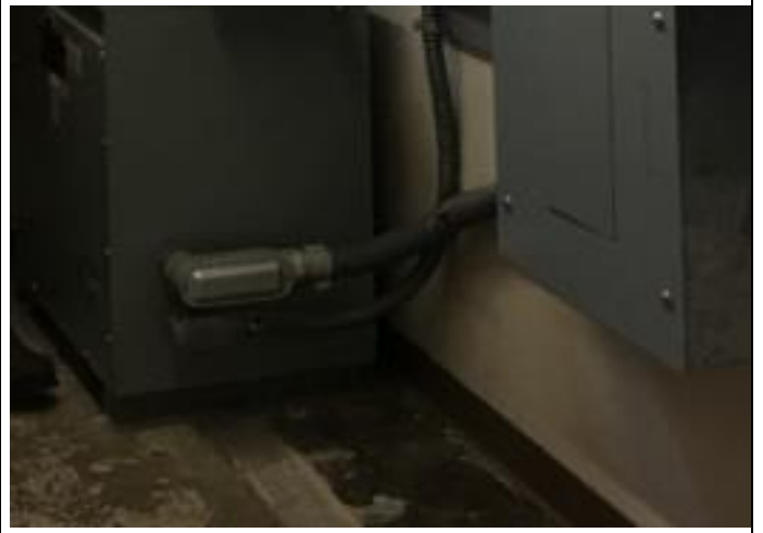
PHOTO 44 Black Mastic – D-20 5% Chrysotile
