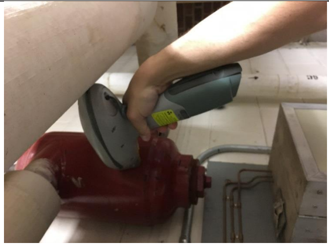
PHOTO 8 Red Painted Mixing Chamber – Below Grade Mech. Room <1mg/cm 2 lead
