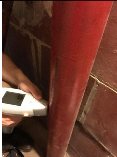
PHOTO 44 Wall in Rm.360 East Pipechase Tower 3 <1mg/cm 2 lead
