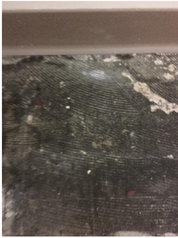
PHOTO 43 Black Mastic – D-20 5% Chrysotile
