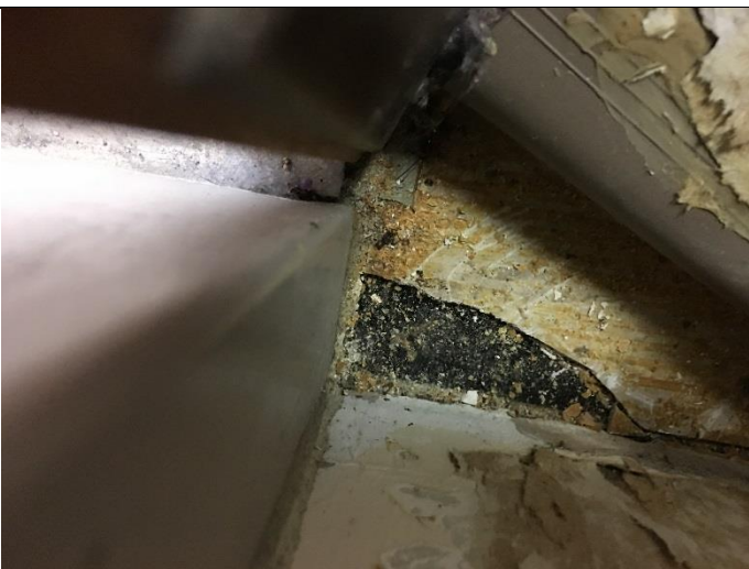
PHOTO 29 Beige VFT Black Mastic (under carpet) – D 21
