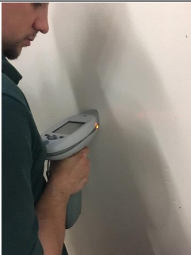
PHOTO 81 East Wall - D-20 <1mg/cm 2 lead
