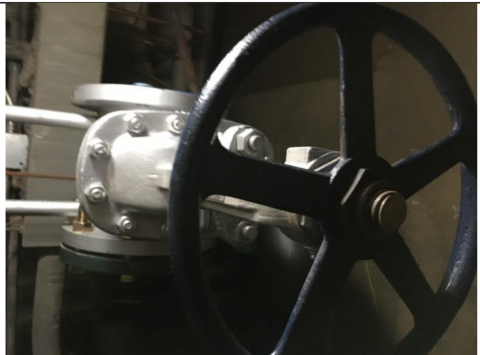
PHOTO 42 Silver Valve - Tunnel <1mg/cm 2 lead
