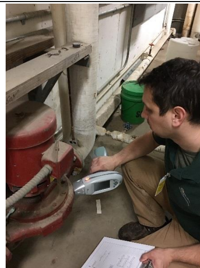
PHOTO 12 Red Painted Valve – Below Grade Mech. Room <1mg/cm 2 lead
