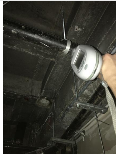
PHOTO 52 Black Pipe D-17 Hallway <1mg/cm 2 lead
