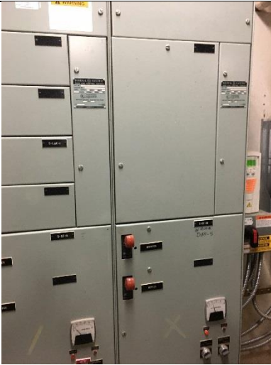
PHOTO 1 Electrical Panel – Below Grade Mechanical Room <1mg/cm 2 lead
