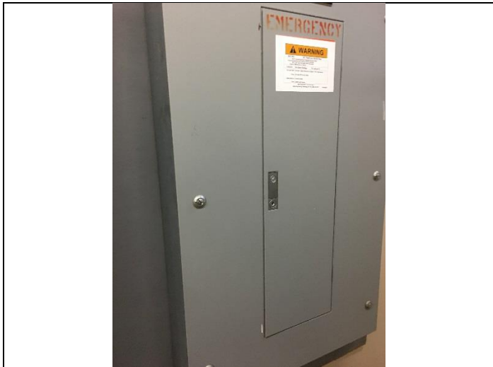
PHOTO 83 Breaker Box – D-20 <1mg/cm 2 lead
