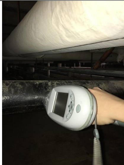
PHOTO 36 Black Pipe – Tunnel <1mg/cm 2 lead
