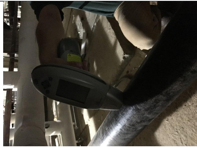
PHOTO 33 Black Pipe – Tunnel <1mg/cm 2 lead
