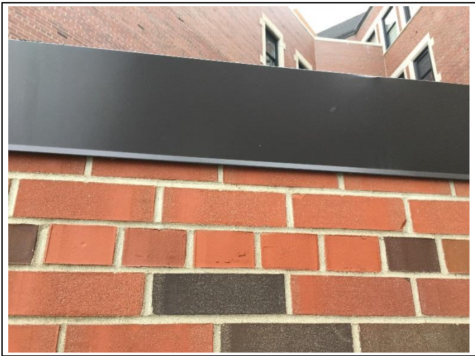
PHOTO 26 Black Flashing - Exterior <1mg/cm 2 lead
