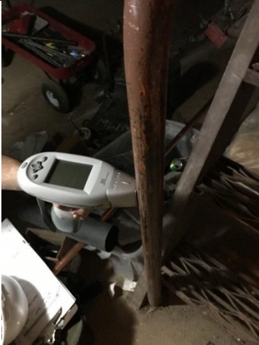
PHOTO 39 Brown Hand Railing-Stairs to Tunnel 3.8 mg/cm 2 lead
