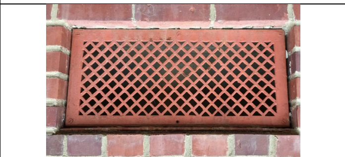
PHOTO 29 Red Decorative Grate on vertical wall - exterior 10.2 mg/cm 2 lead
