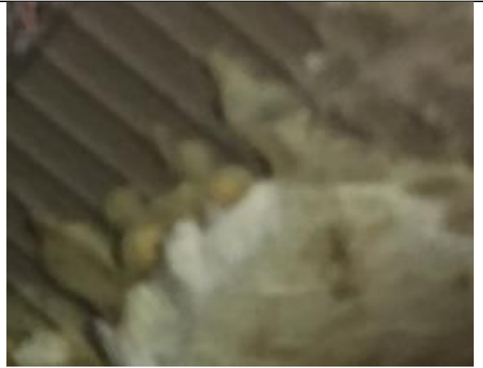
PHOTO 26 Tan Base Cove Mastic
