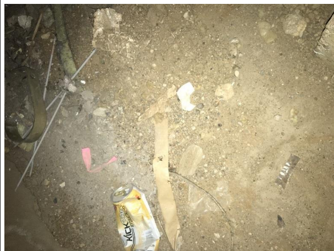
PHOTO 17 Debris on Tunnel Floor
