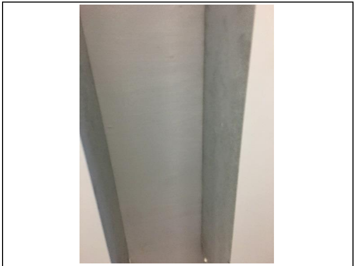
PHOTO 84 Panel behind Breaker Box – D-20 <1mg/cm 2 lead
