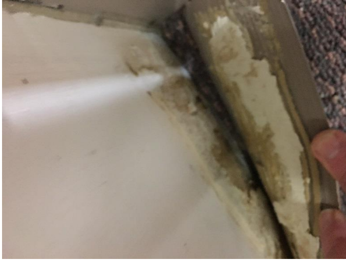
PHOTO 25 | Tan Base Cove Mastic
