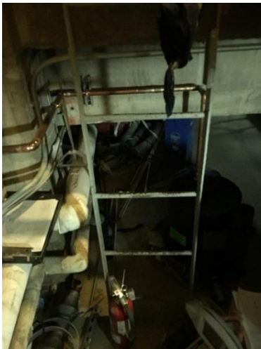
PHOTO 41 Gray ladder in Tunnel 3.1 mg/cm 2 lead
