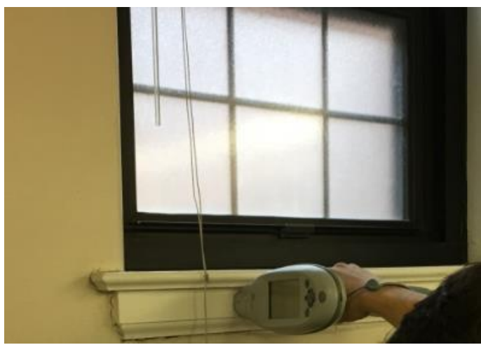
PHOTO 71 Window Sill and Trim Below Window 5.3 mg/cm 2 lead
