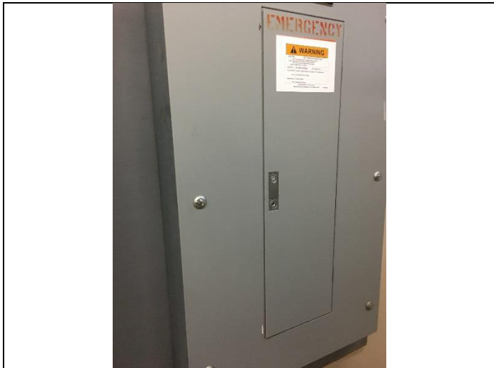
PHOTO 83 Breaker Box – D-20 <1mg/cm 2 lead
