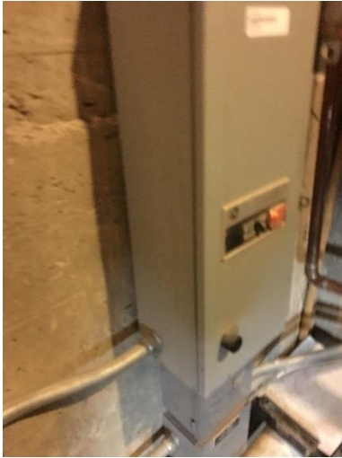
PHOTO 43 Wall in Hallway Tower 3 <1mg/cm 2 lead
