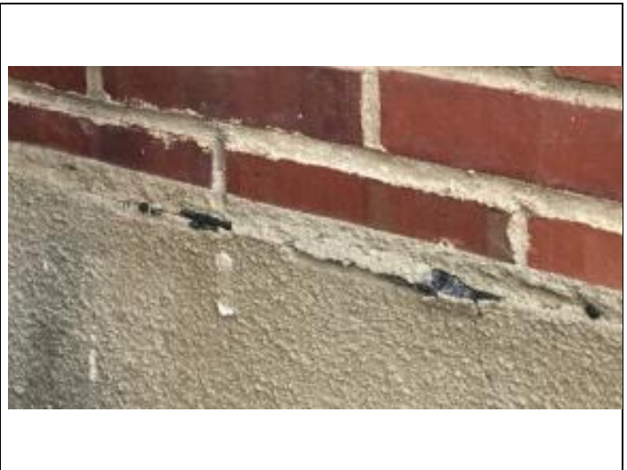
PHOTO 6 | Black Tar Under EFIS – Mech. Room Entry
