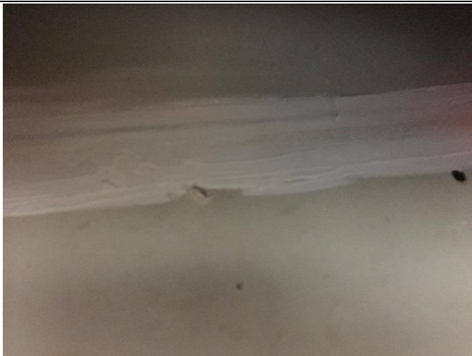
PHOTO 21 | Drywall/Joint Compound D-17
