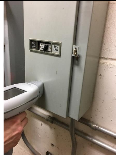
PHOTO 14 Gray Breaker Box – Below Grade Mech. Room <math><1\text{mg}/\text{cm}^2\text{ lead}</math>
