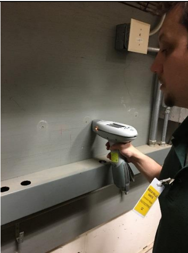
PHOTO 9 Gray Painted Wood Panel – Below Grade Mechanical Room <math><1\text{mg}/\text{cm}^2</math> lead
