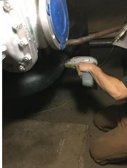
PHOTO 38 Black Pipe – Tunnel <1mg/cm 2 lead
