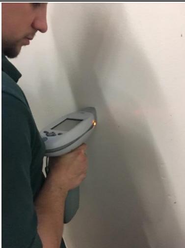
PHOTO 81 East Wall - D-20 <1mg/cm 2 lead
