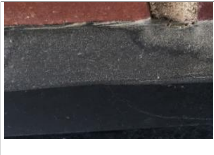
PHOTO 11 Gray Window Caulk - Exterior
