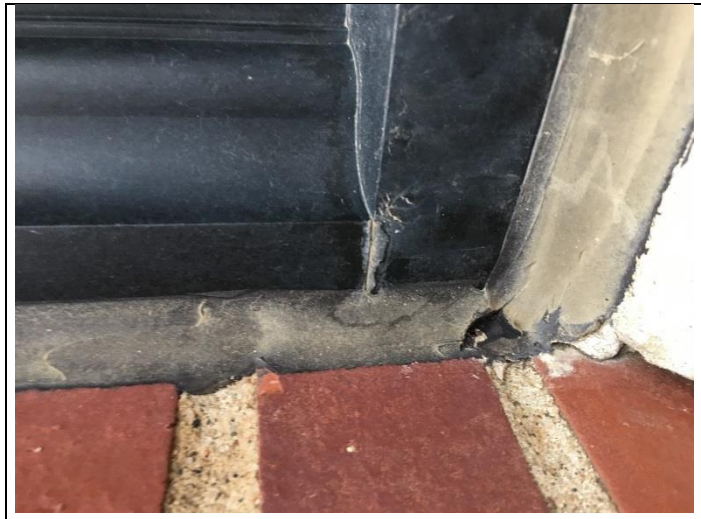
PHOTO 10 Gray Window Caulk - Exterior
