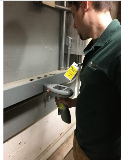
PHOTO 10 Gray Painted Casing – Below Grade Mechanical Room <math><1\text{mg}/\text{cm}^2</math> lead
