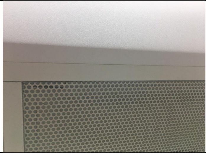
PHOTO 55 Ceiling Grid Hallway by D-17 <1mg/cm 2 lead
