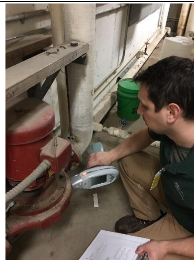
PHOTO 12 Red Painted Valve – Below Grade Mech. Room <math><1\text{mg}/\text{cm}^2</math> lead
