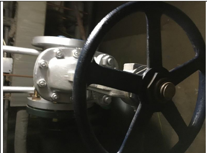
PHOTO 42 Silver Valve - Tunnel <1mg/cm 2 lead
