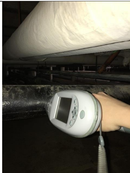
PHOTO 36 Black Pipe – Tunnel <1mg/cm 2 lead
