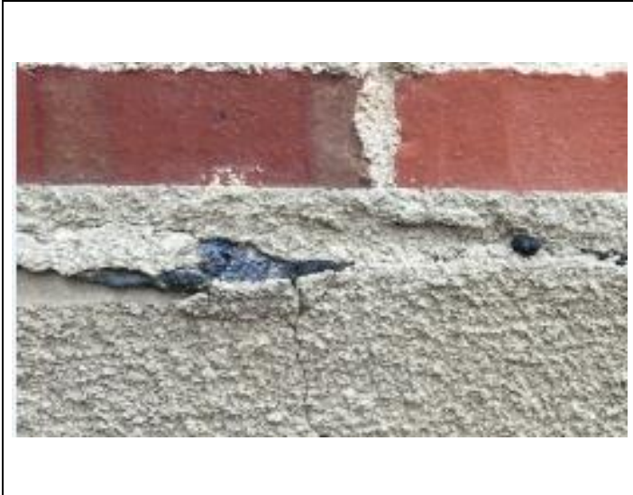
PHOTO 7 Black Tar Under EFIS – Mech. Room Entry
