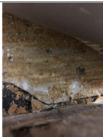
PHOTO 30 | Beige VFT Black Mastic (under carpet) – D 21
