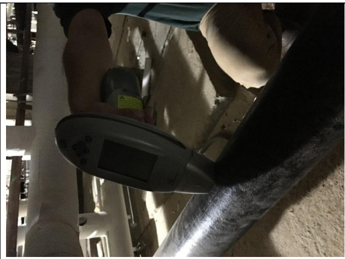
PHOTO 33 Black Pipe – Tunnel <1mg/cm 2 lead
