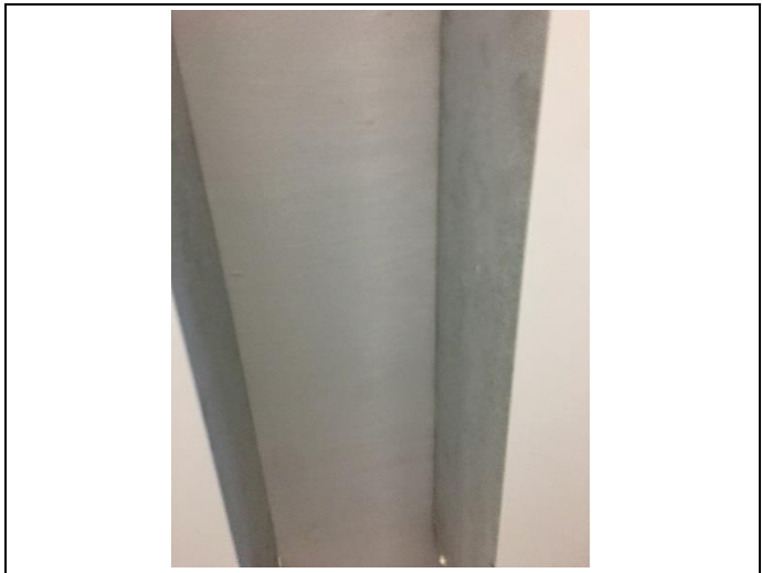
PHOTO 84 Panel behind Breaker Box – D-20 <1mg/cm 2 lead
