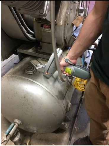
PHOTO 7 Silver Painted Tank – Below Grade Mech. Room <math><1\text{mg}/\text{cm}^2</math> lead
