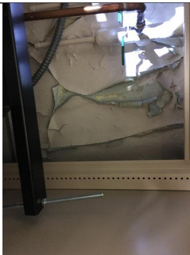
PHOTO 75 Peeling White Paint Under Sink <1mg/cm 2 lead
