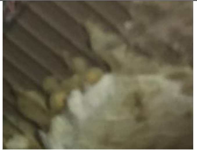
PHOTO 26 | Tan Base Cove Mastic
