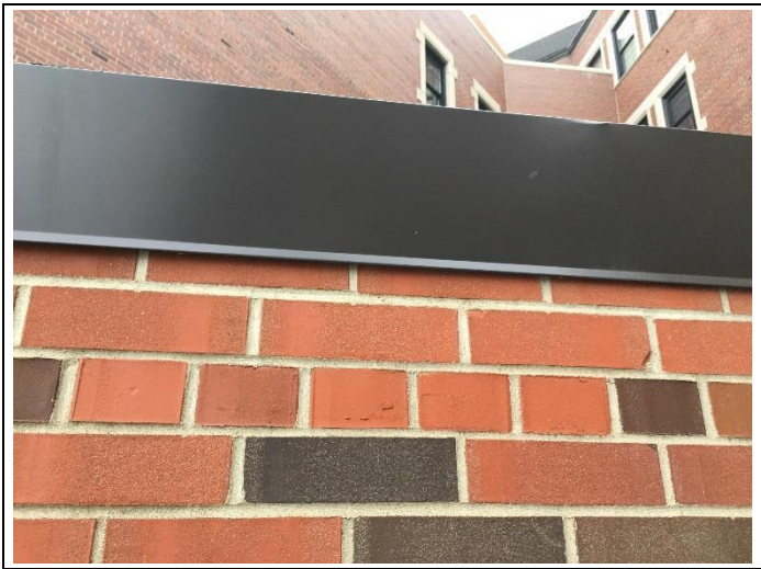
PHOTO 26 Black Flashing - Exterior <1mg/cm 2 lead
