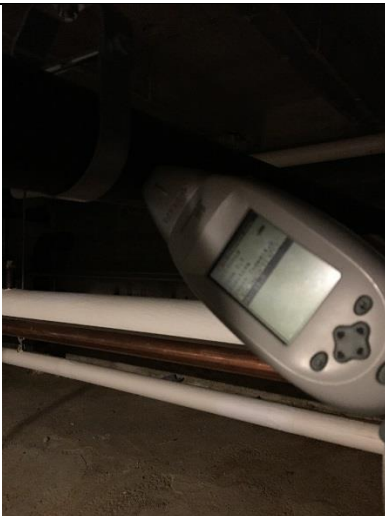
PHOTO 35 Black Pipe – Tunnel <1mg/cm 2 lead
