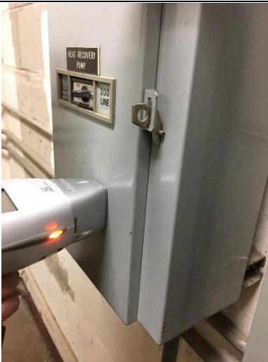
PHOTO 13 Gray Breaker Box – Below Grade Mech. Room <math><1\text{mg}/\text{cm}^2\text{ lead}</math>
