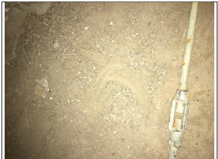
PHOTO 16 Debris on Tunnel Floor
