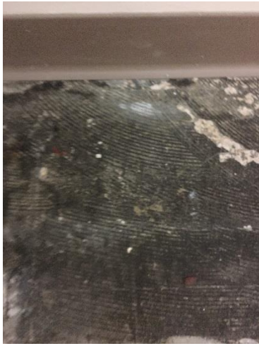
PHOTO 43 Black Mastic – D-20 5% Chrysotile
