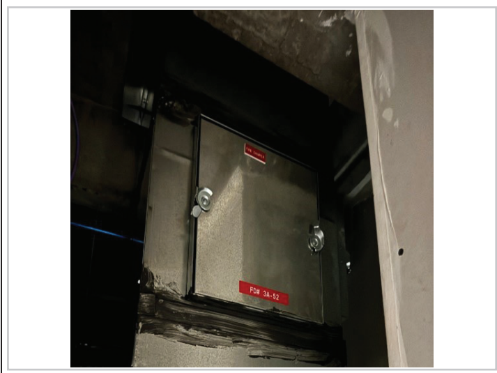
Picture of Damper Tag / Equipment
