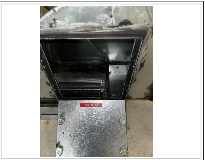
Picture of Damper Re-Opened
