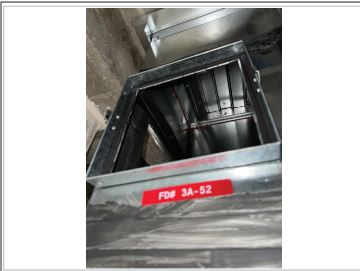
Picture of Damper Closed
