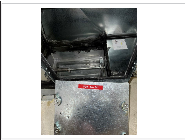
Picture of Damper Closed
