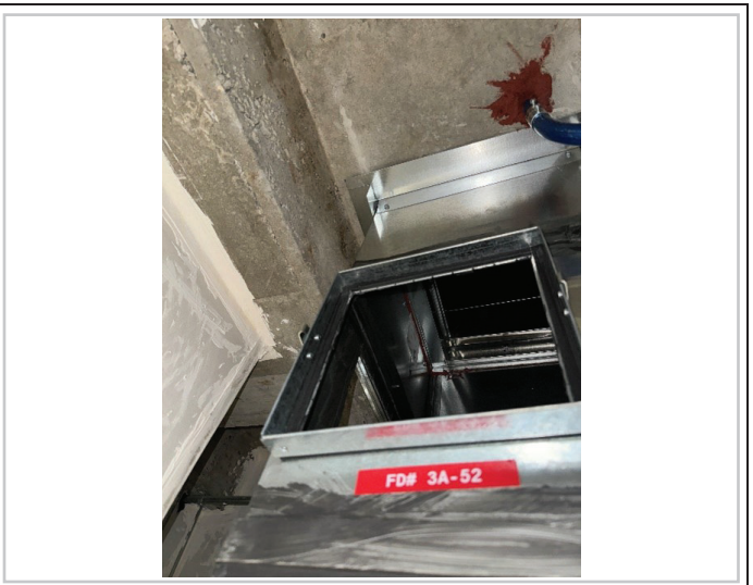
Picture of Damper Re-Opened
