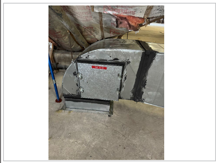
Picture of Damper Tag / Equipment
